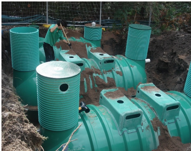
The InnoFlow/Orenco fibreglass primary and recirculation tanks being installed in June 2010 by Kerry Flanagan Wastewater
